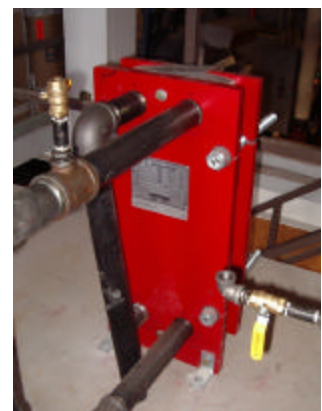
Figure 6 District Energy Heat Exchanger
