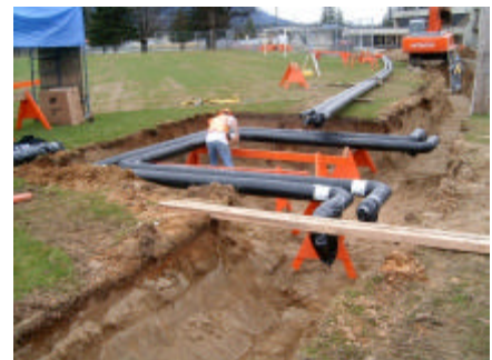
Figure 3 District Energy Piping 3
